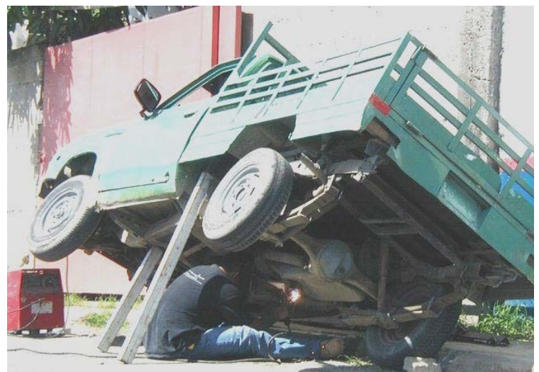
It's fairly obvious that a 'risk management' approach wasn't applied to this job. The third place-getter in Absolute Shocker and Bodgey Scaffold of the Year 2004 (WorkSafe Victoria 'Award')
