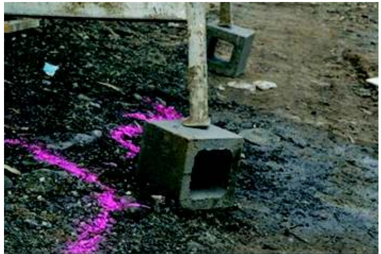
The genius that erected this scaffold will be subject to uniform regulations when WHS harmonisation is in place across Australia in 2012.
