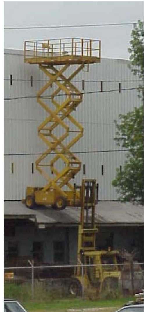
Clearly not a recommended use for forklifts. Photo of "second place getter" in WorkSafe Victoria's "Absolute Shocker and Bodgey Scaffold of the Year" Award 2004.
